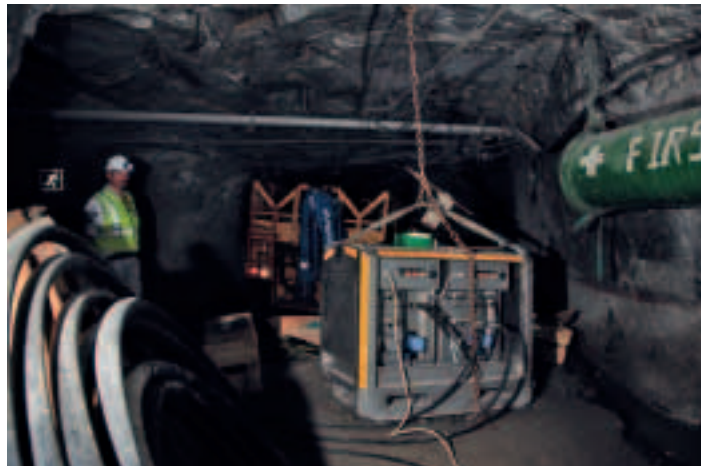
Peterstow power pack underground - compact and efficient
